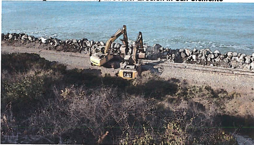
Figure 4. Track Repairs After Erosion in San Clemente
