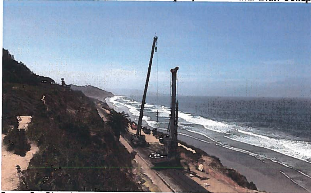
Figure 3. Trackside View of the February 28, 2021 Del Mar Bluff Collapse
